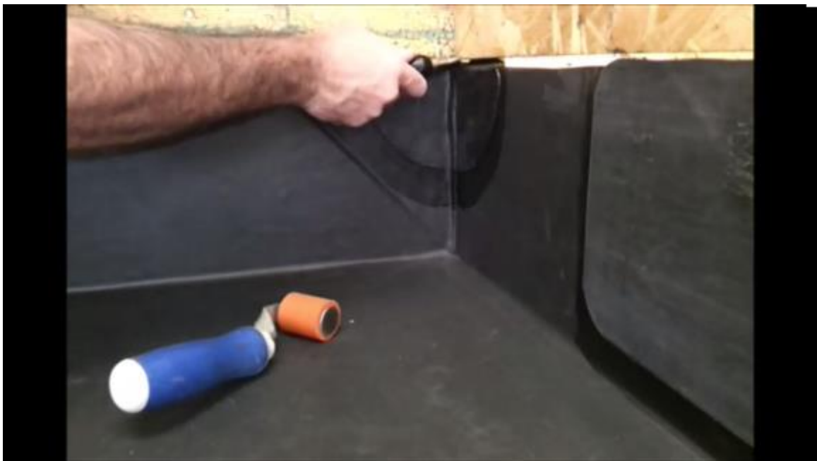
Fig 4: Using the penny roller to make the seal on the top edge.
